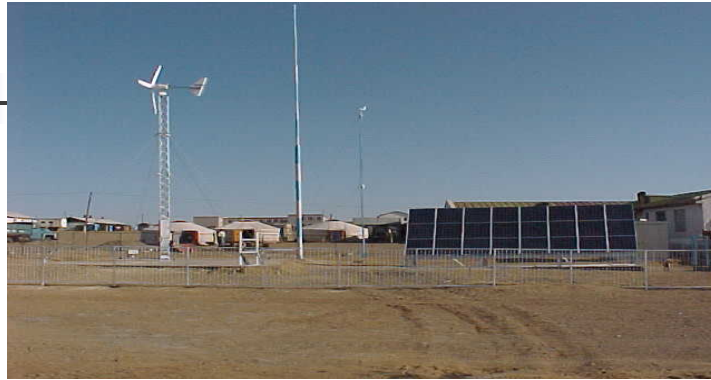
The PV-Wind hybrid system at Tariat soum, Atkhangai aimag, installed under JICA project (Japan)
