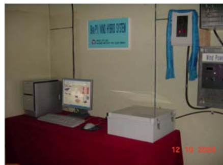
Data acquisition system
