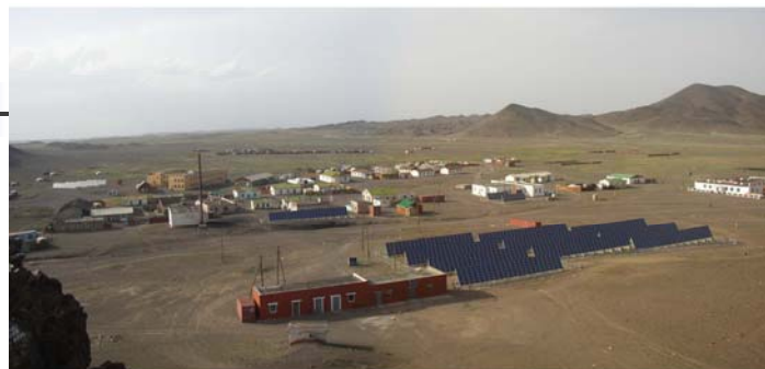
200 kW PV-Diesel hybrid system at Noyon soum installed under NEDO Research project The demonstrative research project on dispersed type PV power generation system in Mongolia
